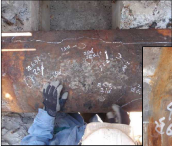
Photo: Corroded Pipe after dismantling retaining wall
