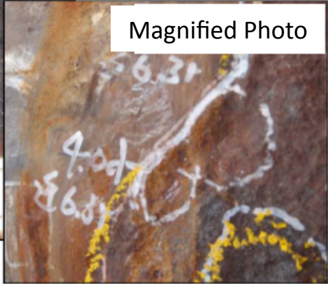
Nominal Thickness 6.5mm Max. Corrosion Depth: 4mm
